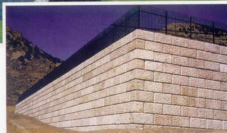
Nevada D.O.T. Maintenance Yard Virginia City, NV. Quarry Stone, MSE wall built to expand storage area.
